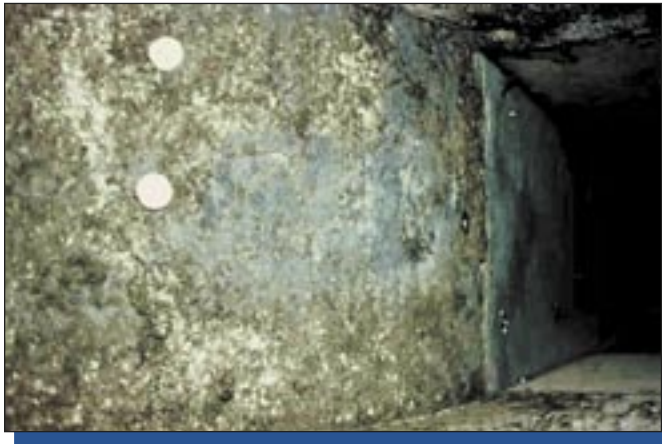
Prior to application of Foster® 40-20™ coating, fungal wipe samples on the fibrous glass duct liner showed average fungal levels of 45,000 colony forming units per square centimeter (cfu/cm2).
